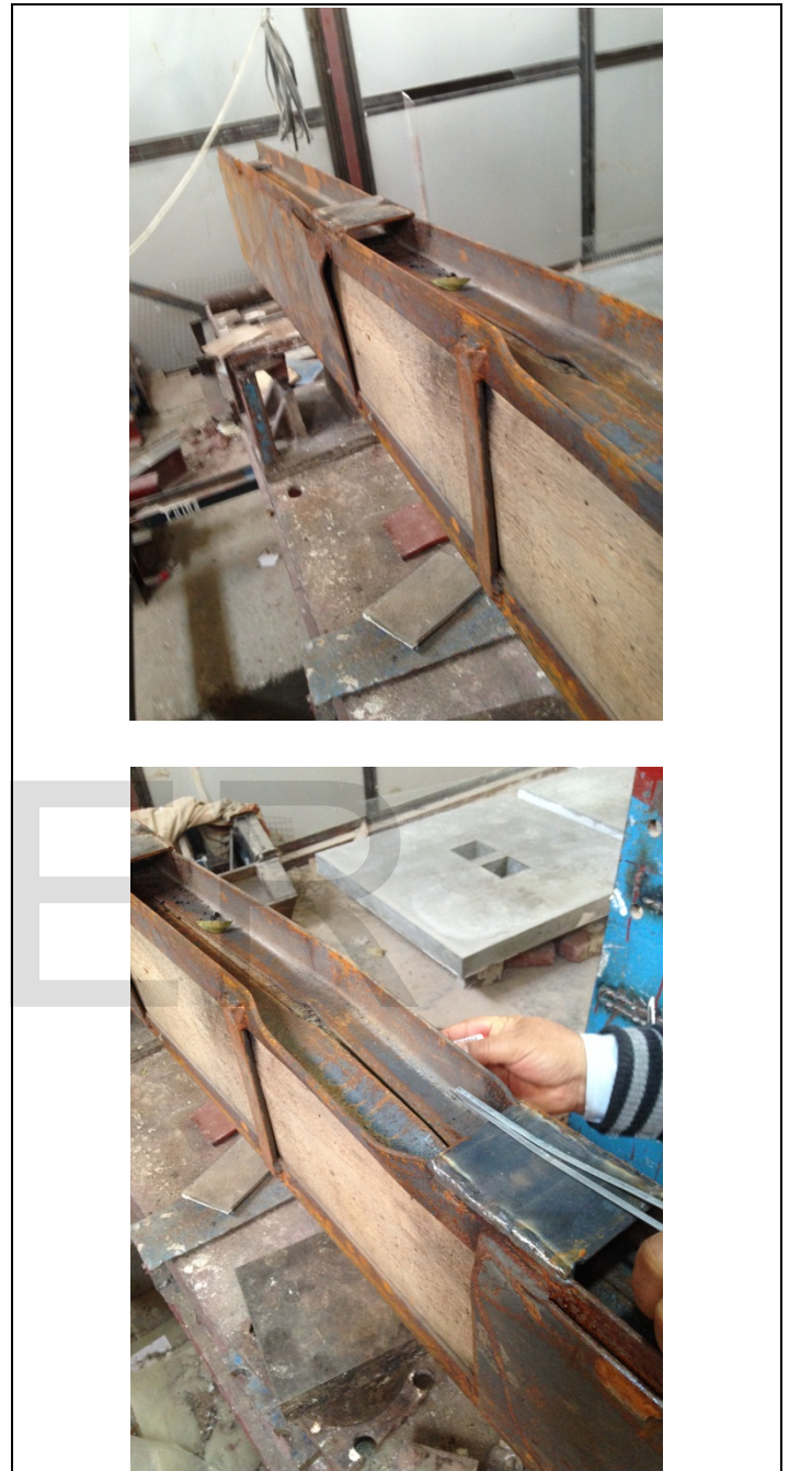
Fig. 8. Local Buckling in Angles and tying plates
